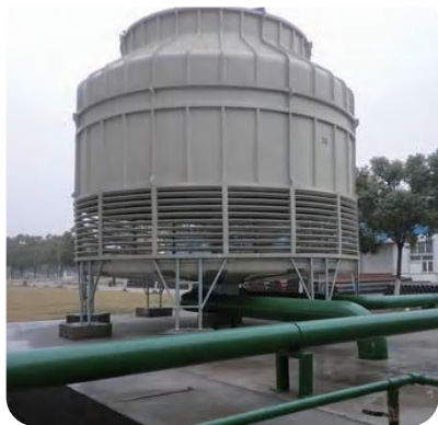
Condensing tower seal
