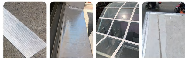
Roof crack Window sill gap Glass room joints Top of carriage
