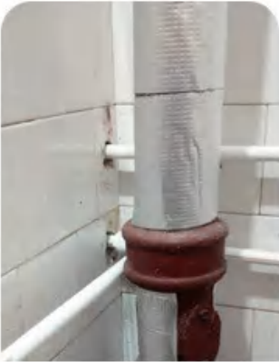
No pressure sewer pipe
