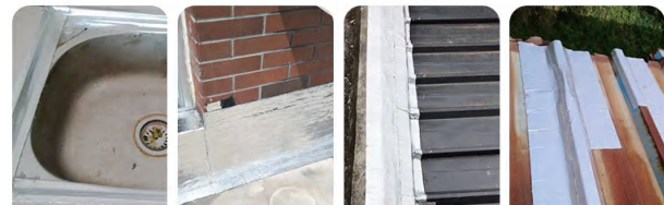
Dish washing sink Gap between wall and ground Color steel and wall joints Color steel tile gap
